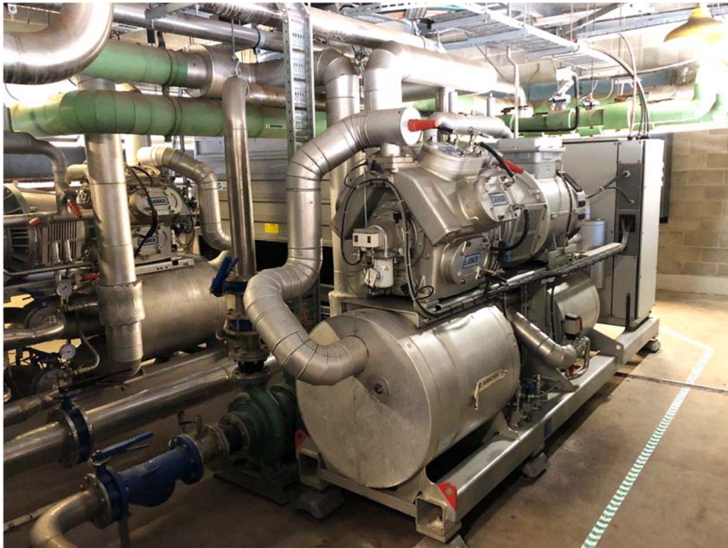
Figure 5. Plant room interior showing two chillers and a cooling tower in the background.
